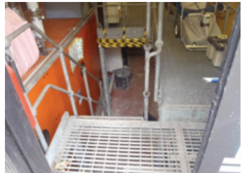
The example picture here shows a very restricted plantroom at the famous Hurlingham Club where we carried out extensive works on the swimming pool plant.
