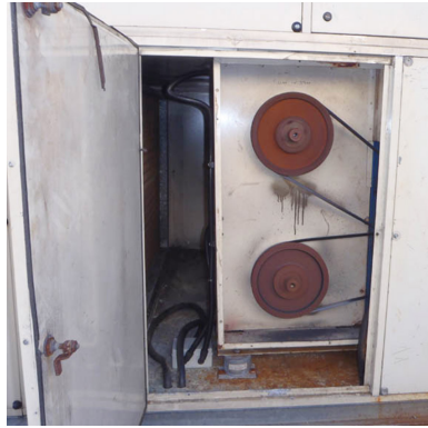
Before - inefficient belt driven fans
