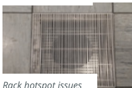
Rack hotspot issues
