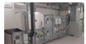
HTM 03-01 compliant AHU
