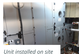
Unit installed on site
