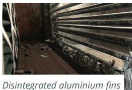
Disintegrated aluminium fins
